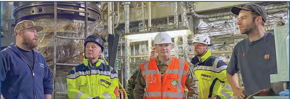
MV Endurance Chief Engineer TJ Lumb provided a briefing and tour of the engine room.
